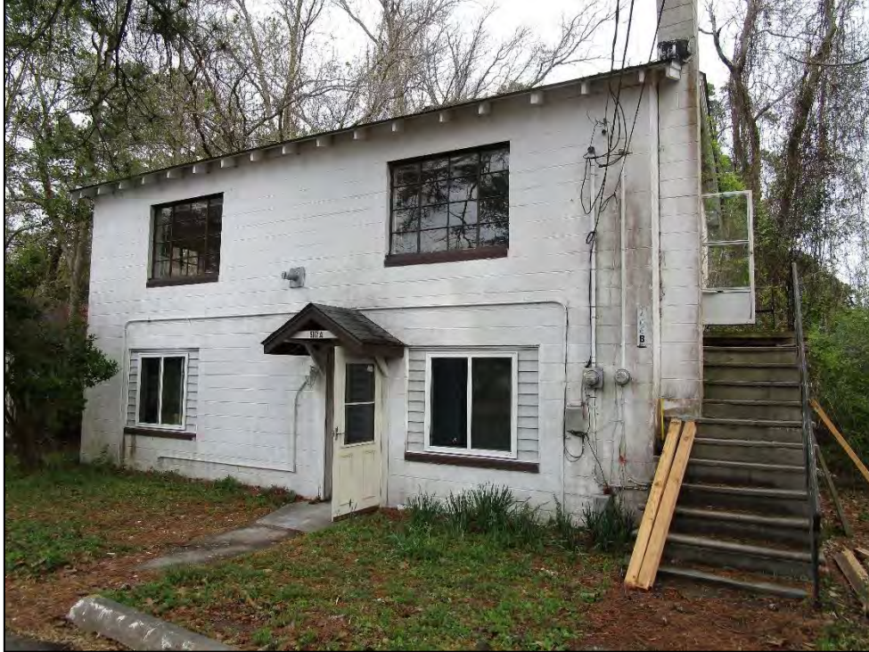
Jesse Trader House, Apartment Building (1950) façade (south facing), view to the northwest.
