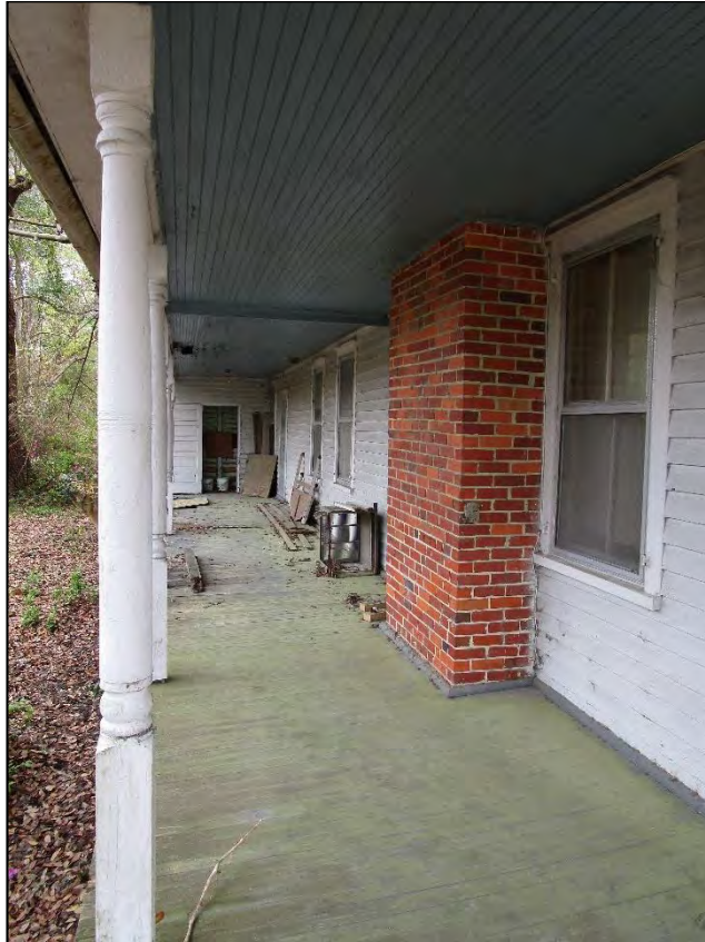
Jesse Trader House porch detail; view to the north along the west elevation. Note the exterior closet addition at the end of the porch.
