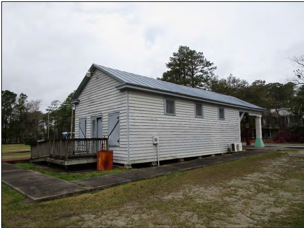
Hugh Trader Store, oblique view of the rear (south) and east elevations, view to the northwest
